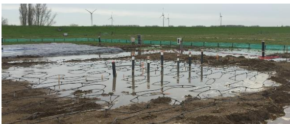
Figure 5 – Beaudrain-S section with monitoring equipment (after some days of consolidation).
