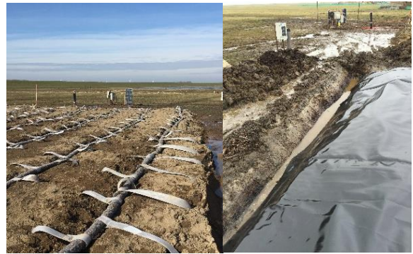
Figure 3 – Traditional liner vacuum system, left: vertical drains connected to the horizontal drains, right: liner in trench surrounding the area.
