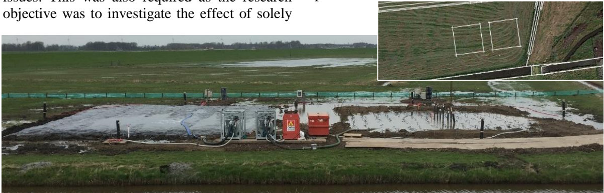
Figure 2 – Trial area with the traditional vacuum system (left) & the Beudrain-S system (right)
